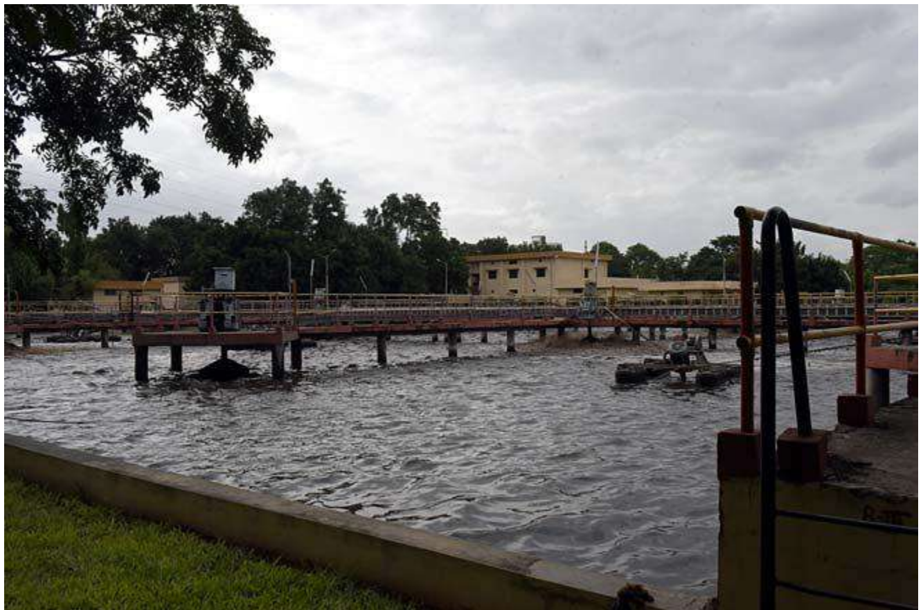
Water & Sewage Treatment Plant, Nagole
