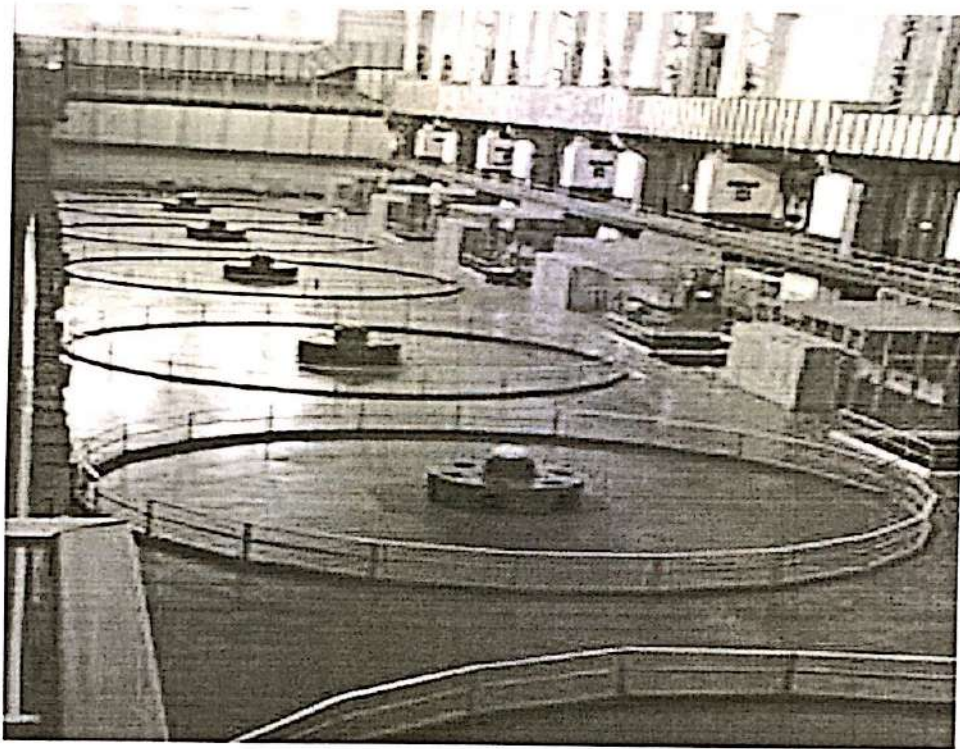
Turbines of power House
